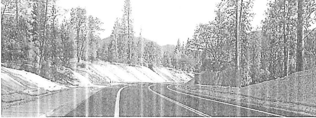
Lance Gulch Road behind the Mill looking south just prior to opening, October 2015
