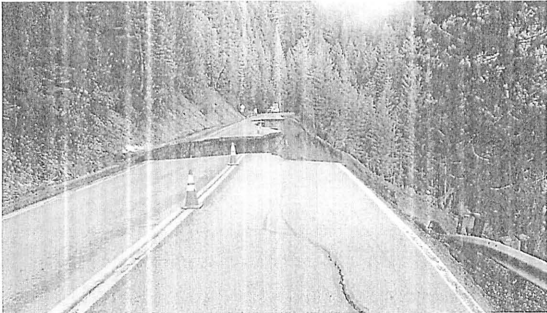
State Highway 3 at Slate Creek, March 2016
