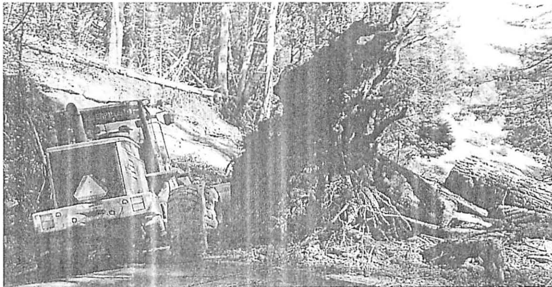
Denny Road PM 21, 2016 Winter Storm Damage
