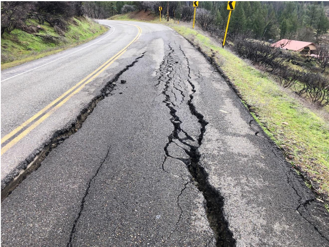
Mad River Road failure, shift 4-6 in. high, cracks 4-6 in. wide and 18-20 in. deep
