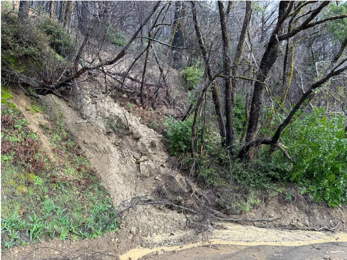
Long Ridge Road slide in Kettenpom
