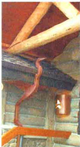
Choose good materials and avoid polluting ones (like this copper downspout)
