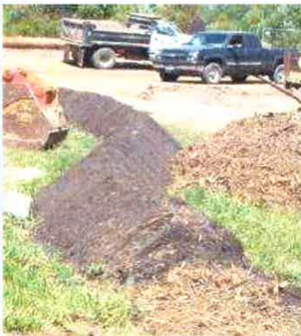
This berm, made of compost instead of ordinary loose soil, is highly effective at reducing sediment transport off-site and can be installed by hand or machine
