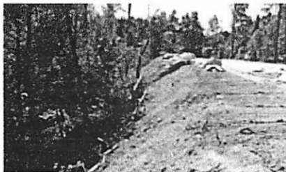
Unstable fill slopes along the .7 acre grow pad. (The Willits News)
